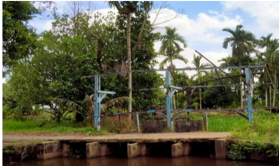
Fig. 4 Condition of the floodgates in the catchment area Parit Keladi 1 (Research, 2022)
