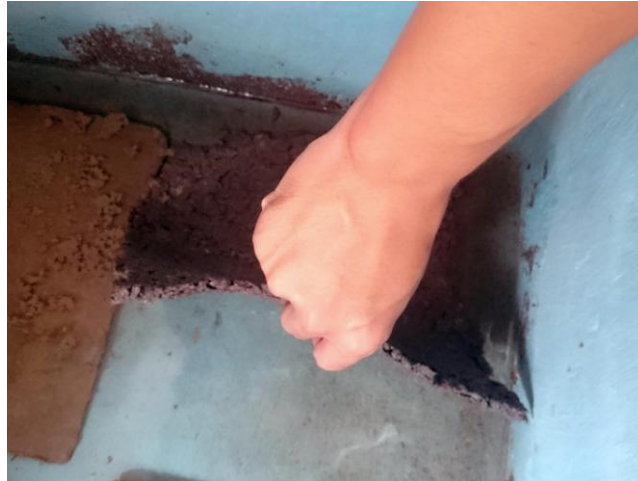
Figure 2. Complete Damage of 0.5 cm Thickness Recycled Paper Panel Source: Author's Documentation, 2016
